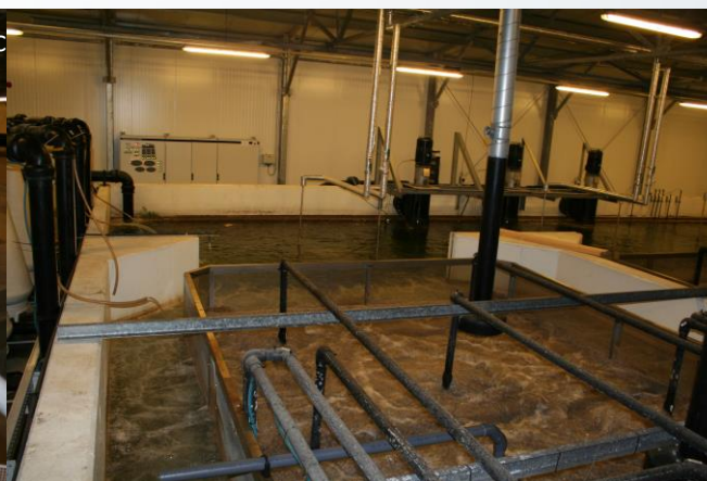
RAS anlegg Grieg Seafood Adamselv © Jelena Kolarevic
