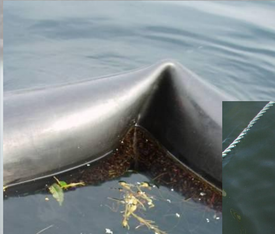
Permanent kinking of the HDPE pipe
