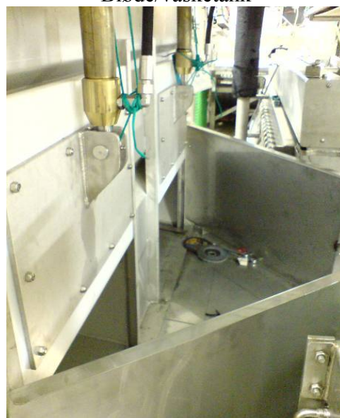
Grader binger (installert 2)
